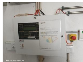
Fire control panel.jpg
