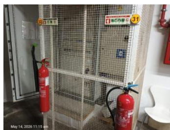
Electrical sub distribution board 2.jpg
