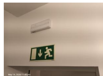
Exit sign and emergency exit.jpg
