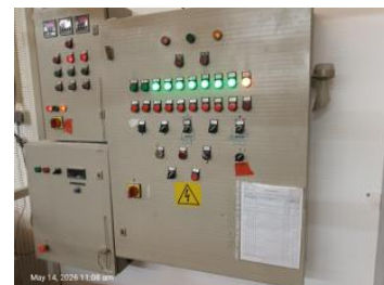
Electrical sub distribution board.jpg
