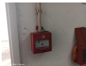
Fire alarm call point_Candle.jpg
