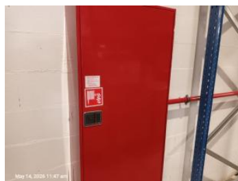
Fire hose reel_Cosmetics.jpg
