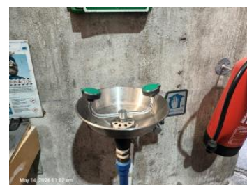
Eye washing station.jpg
