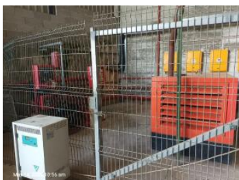
Fire hydrant pump.jpg
